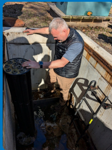
John Pedrick, Contech Engineered Solutions, inspects Jellyfish Filter cartridges at the Treatment Train site in Roger Williams Park.
